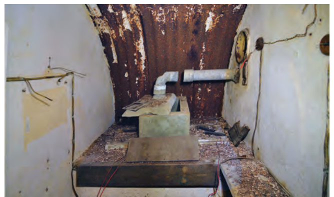
Exhaust box for generators. Photo Chris Warren
